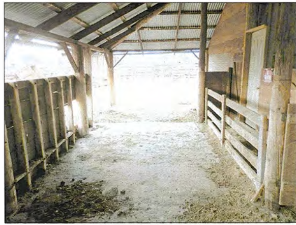
EAST SIDE UTILITY ISLE LOOKING SOUTH (P1 S4.3)
