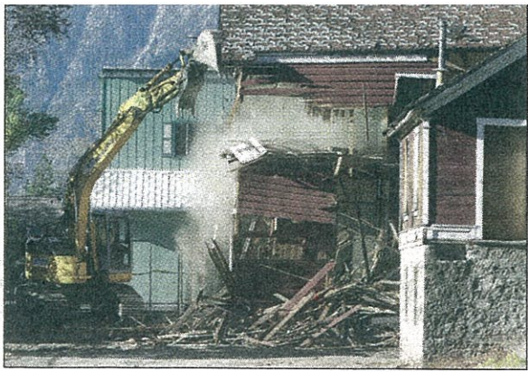
An excavator is used to demolish the historic East Fork Hotel on Monday morning.
