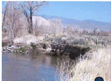
River Bank failure in Dayton Photo by: Ed James
