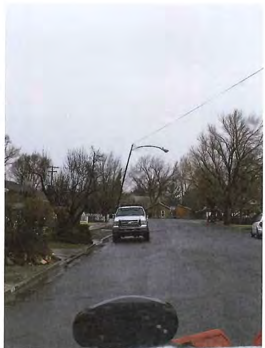
Meadow Lane - Tree Down Pulling over street light NV Energy Notified
