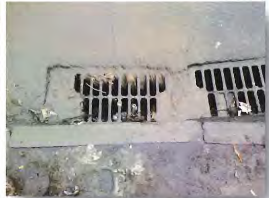
Polluted Stormwater Entering Storm Drain
