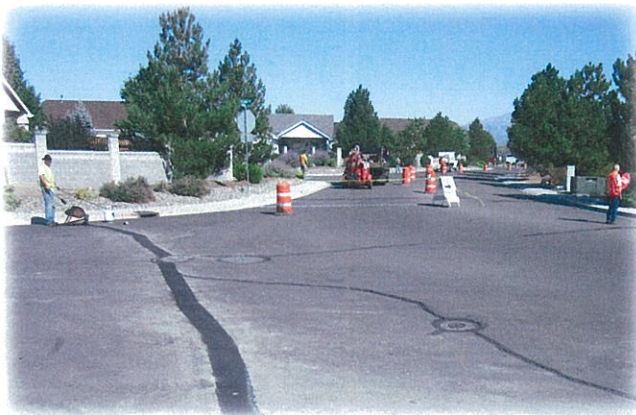
2012 CHICHESTER CRACK PATCH
