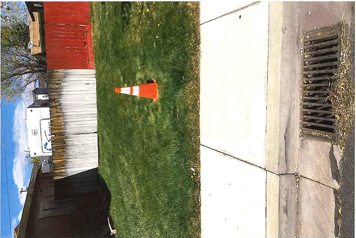
SINKHOLE 10' FROM DE
